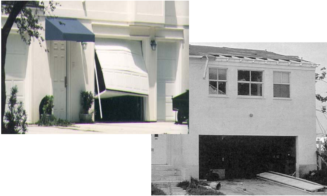
Figure 1-9. Garage Door Performance
