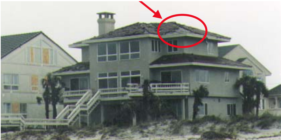
Figure 1-2. Loss of Roof Covering Leads to Interior Water Damage
