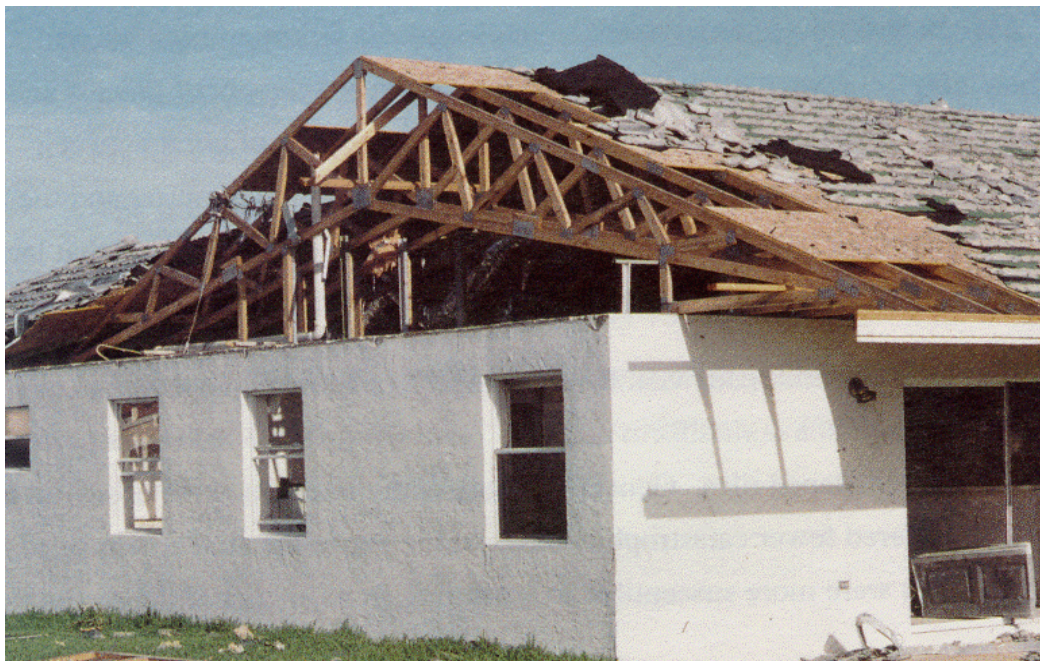
Figure 1-6. Gable End Failure
