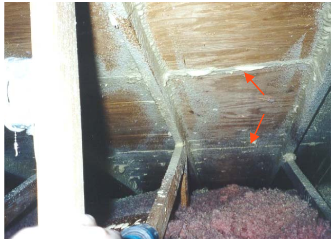
Figure C-2. Sprayed on Structural Adhesives to Seal Plywood Joints (SWR) and Strengthen Roof Deck Attachment
